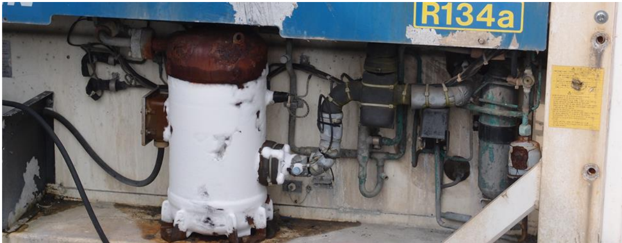
Figure 18. Corrosion on a cooling unit of an old reefer.
